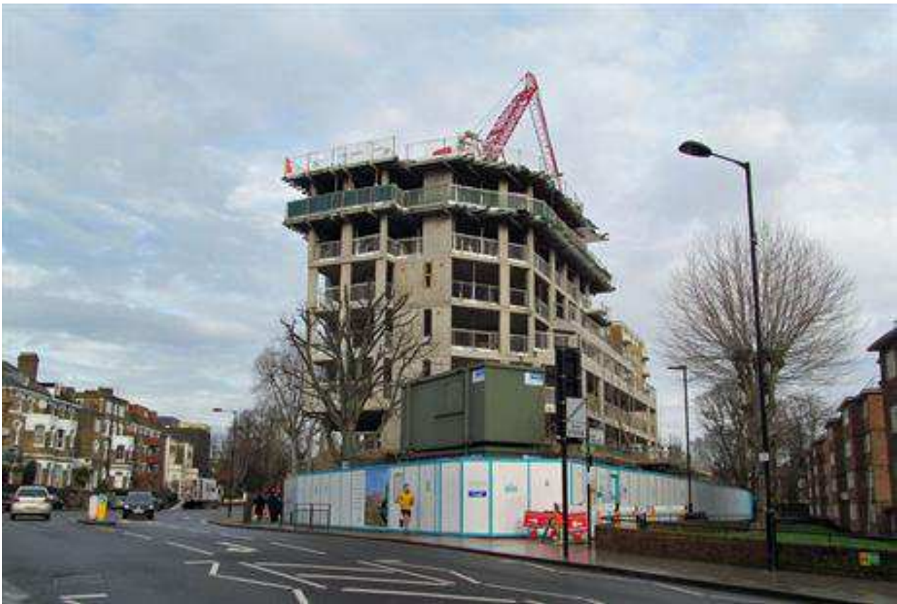
New development: a building site in London. Image by David Holt, Flickr
